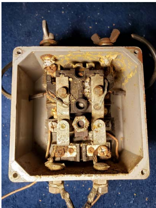
Figure 1. An antenna relay box after 17 years outdoors.
